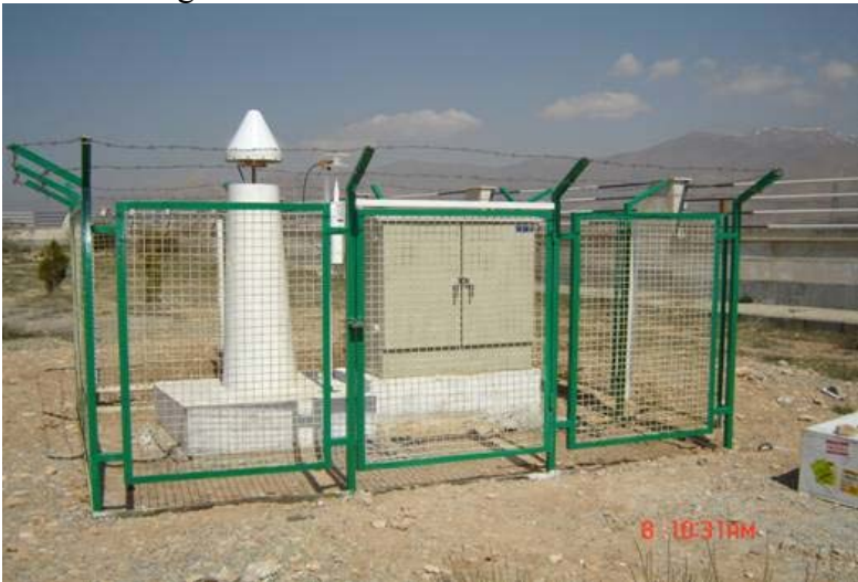
Figure 5: Pillar and rack of HSGD station
